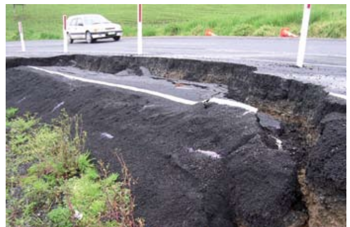
Figure 2. Close up of the slip
