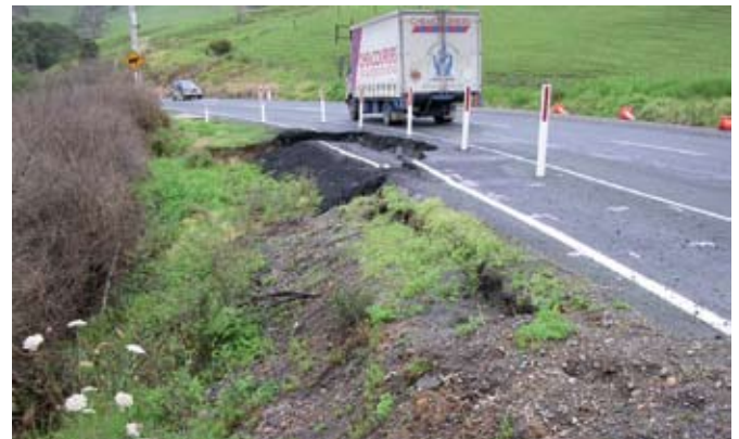
Figure 1. Slip on the shoulder of the road
